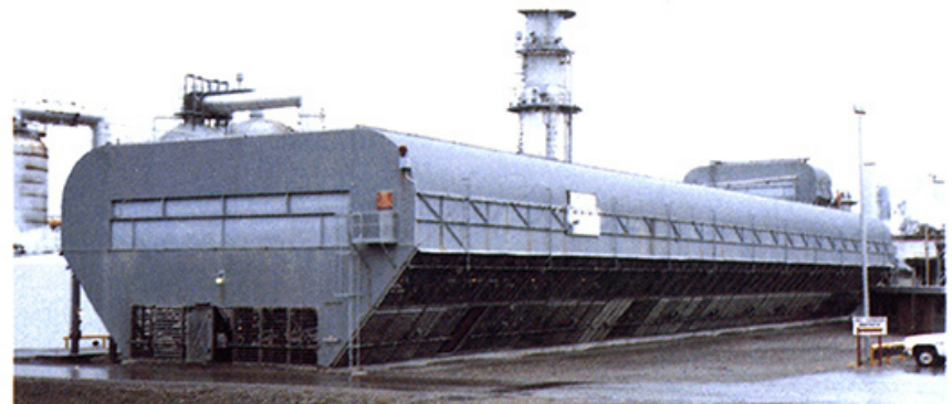
GAS PLANT COOLING UNIT — CANADA
